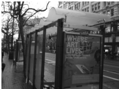
Note missing glass panel.
