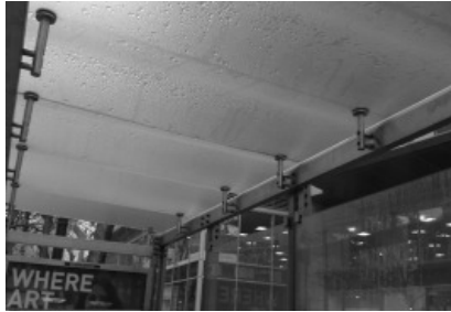
Gaps between roof and walls.
